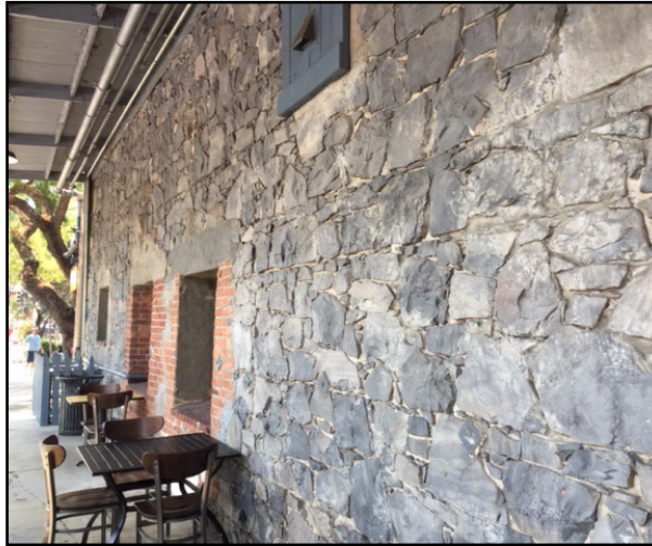
A stone wall of the Great Petaluma Mill, constructed in 1854 by Thom Baylis
