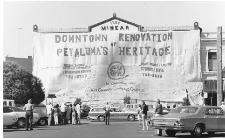
Renovations of Petaluma's McNear Building during the 1970s while preserving its historic architecture
